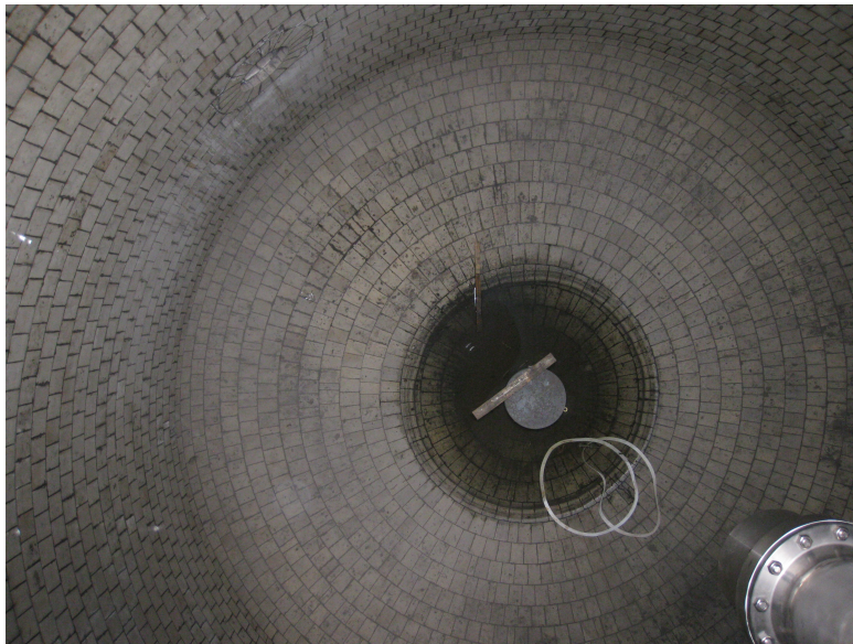
2. Brick lining in an autoclave in metallurgy industry
